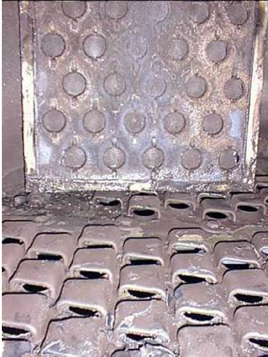
Figure 4. Example of Tray Fouling in Sour Water Stripper Service [13].
