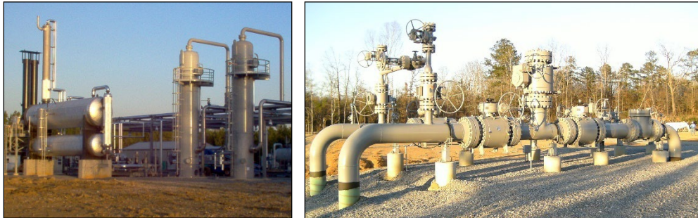
Figure 2. CO 2 Dehydration Unit and CO 2 Pipeline.
